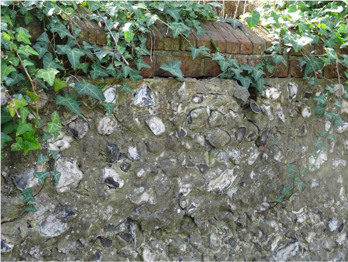
Giles Hill Cemetery Front Wall Spalling
