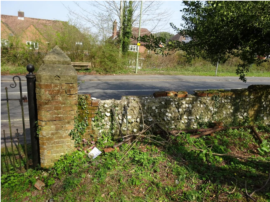
St Giles Hill Cemetery Wall West Damage
