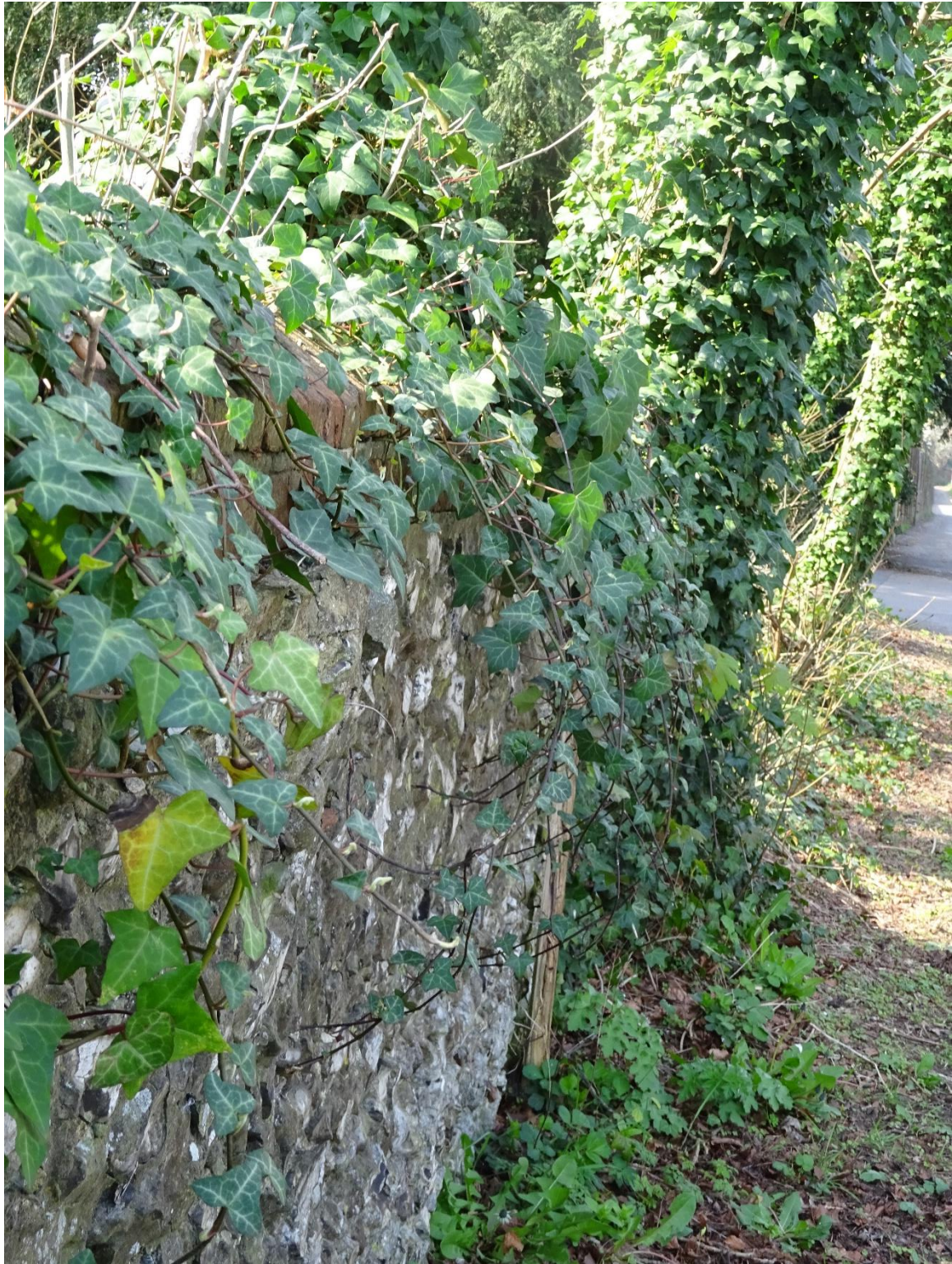
St Giles Hill Cemetery Front Wall West Damage
