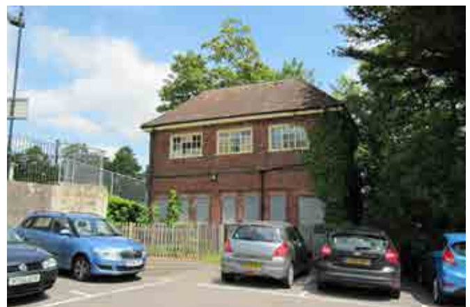
Brick Villa: In state of disrepair with windows boarded shut.
