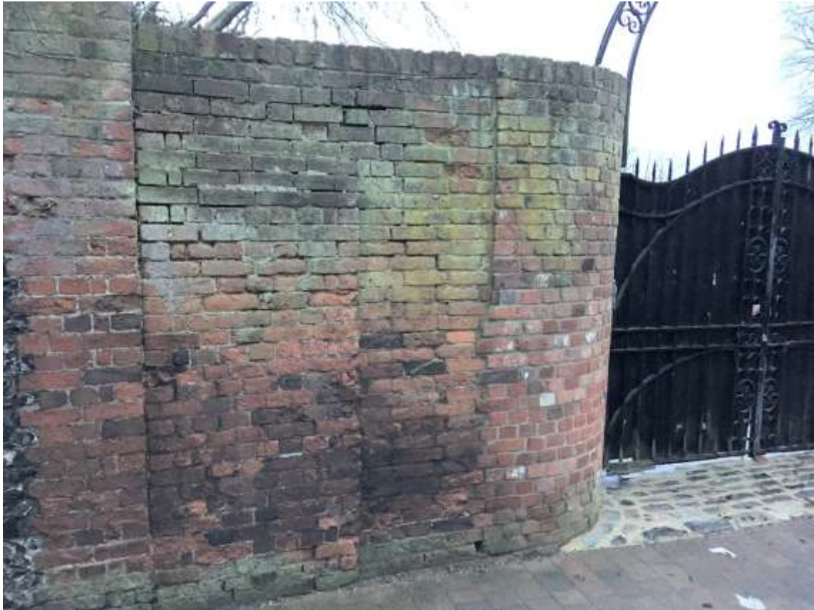
Wall of 13 St Thomas Street 1
